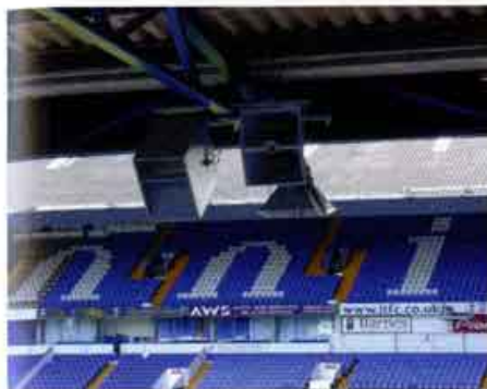
Sophisticated sound systems are not confined to glamorous arenas – this is the Funktion One AX88-based system just installed at Portman Road, Ipswich
