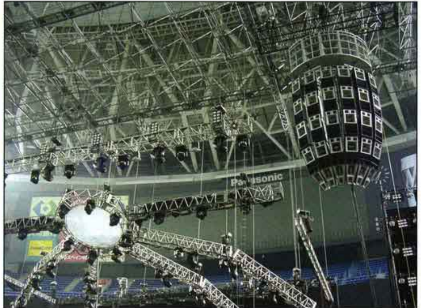
A Funktion-One Resolution speaker cluster being hoisted for a Jamiroquai's concert in Osaka.
